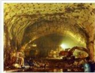
underground storage facilities
